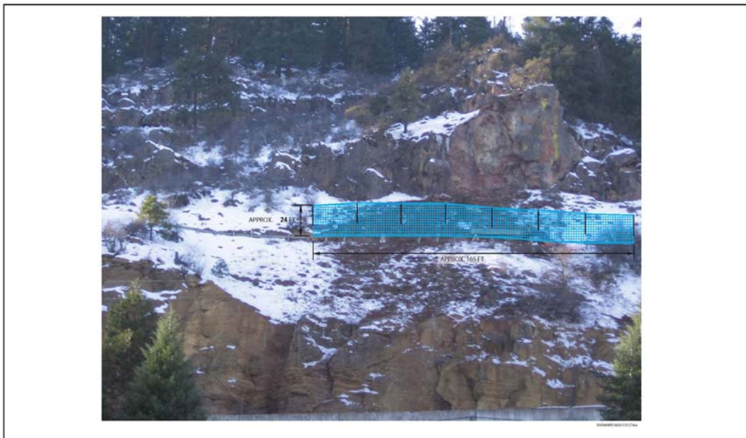
Figure 5 Modified Cable Net Catch Fence
