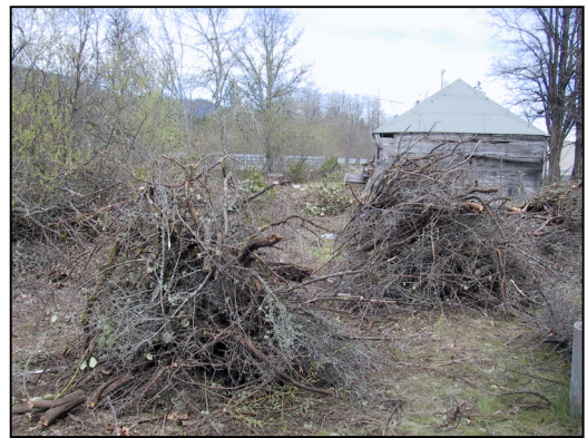
Site C in Selma, Oregon – after treatment. Photo courtesy of the Job Council
