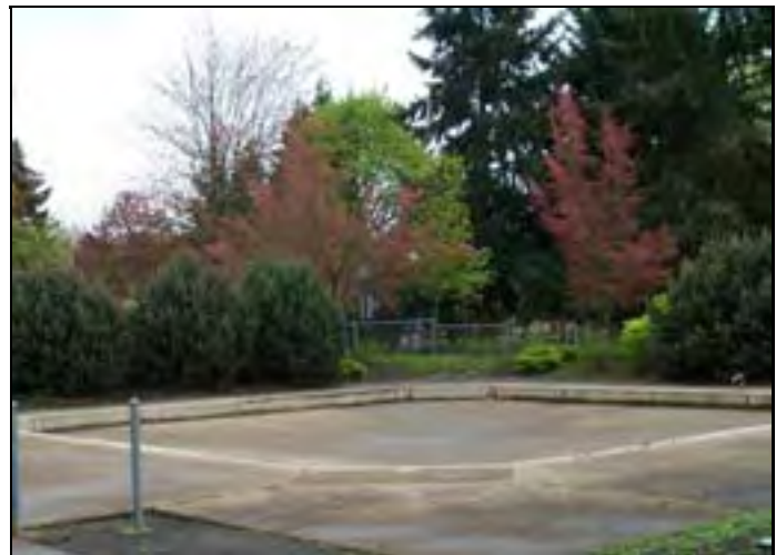
Wading Pools need to be decommissioned per new health standards.
