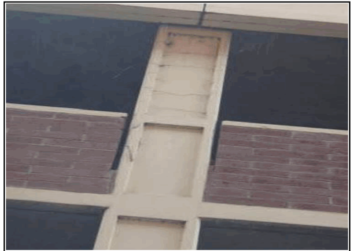
Pearl Street Garage - Spall in Column.
