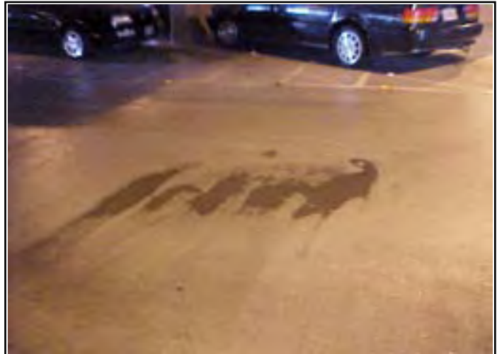
Overpark deck wear
