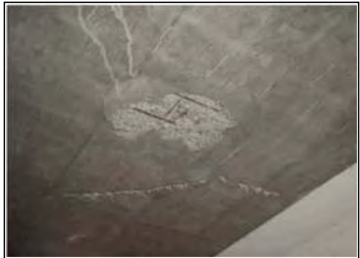
Overpark Garage - Ceiling spalling.
