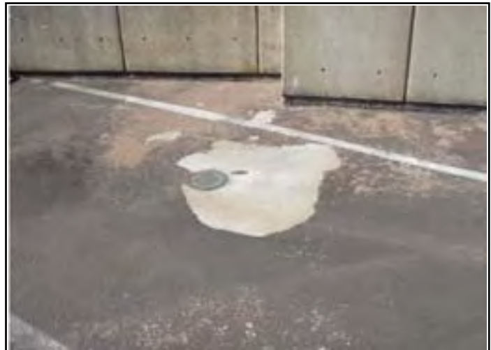
Deteriorated wearing surface on top level
