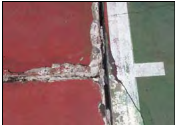
Tennis court surface showing cracking.
