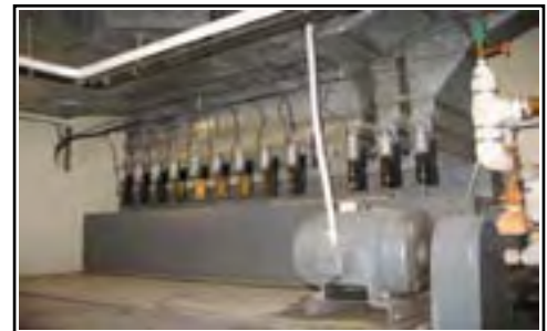
A mechanical room at City Hall.
