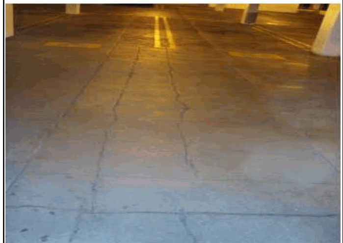
Broadway North Garage - Cracks in pour joint on level P1 from above
