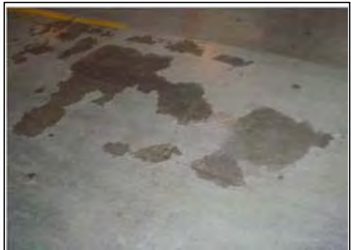
Pearl Street Garage - Deteriorated driving surface above retail space on level 2.
