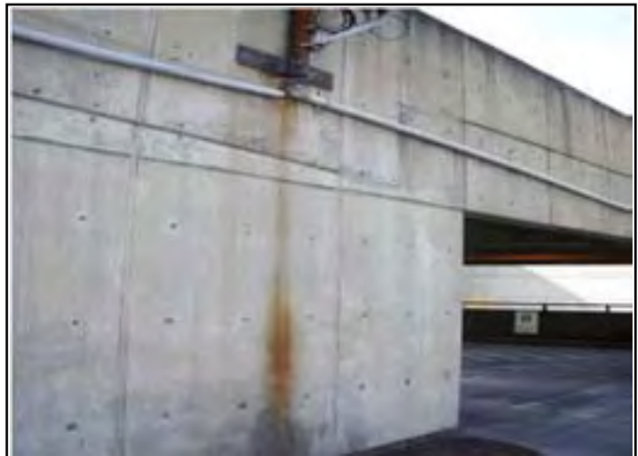
Water leak in wall of Parcade Garage.
