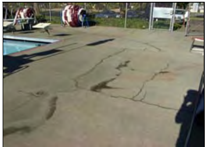
Deteriorating pool deck at Echo Hollow Pool.
