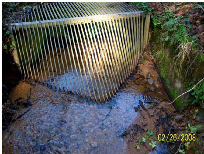
Figure 5. Stormwater drains – Astoria, Oregon
