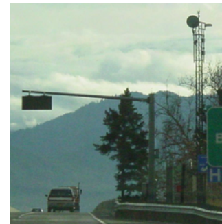
I-5 Weather Station and Overhead Ice Warning Sign
