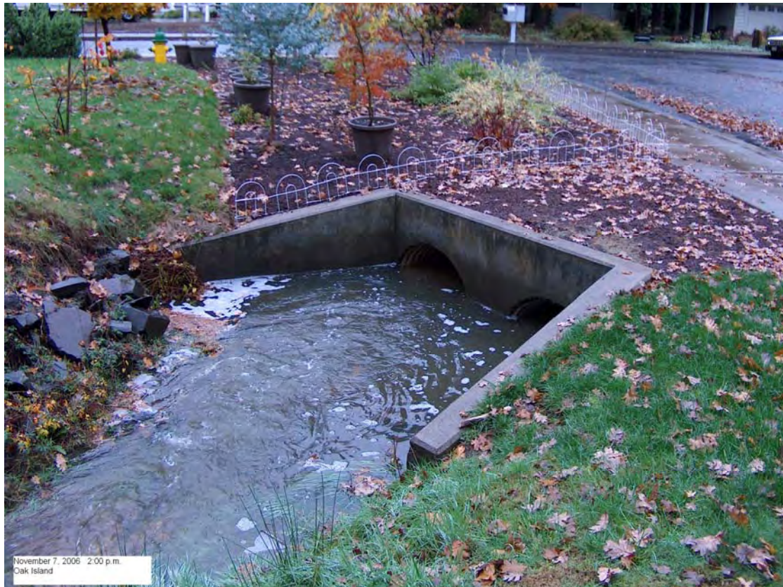
Oak Island Drive Culvert – Estimated depth from crown elevation to WSE is 8".
