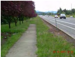
Sidewalk Below Grade
