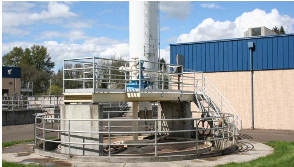
Figure 7-25: Silverton WWTP Dissolve Air Flotation Thickener
