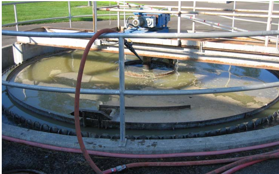
Figure 9-12: Silverton Gravity Thickener
