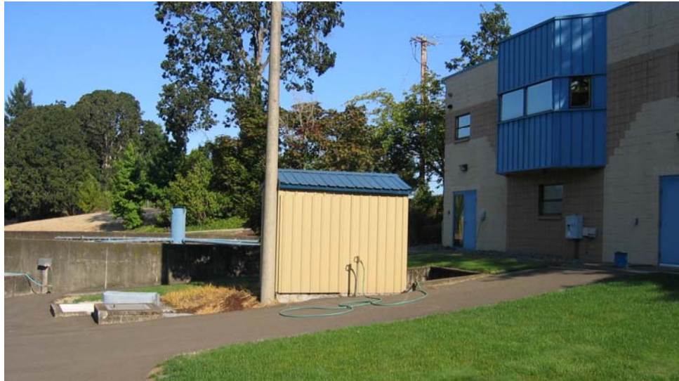
Figure 9-9: Primary Sludge Pump Shelter (Tan Walls with Blue Roof)
