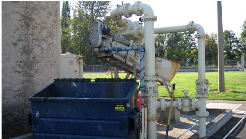
Figure 9-11: Silverton Primary Sludge Degritting Equipment
