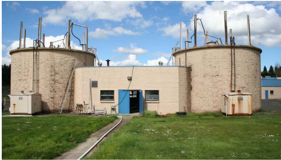
Figure 7-27: Silverton WWTP Anaerobic Digesters
