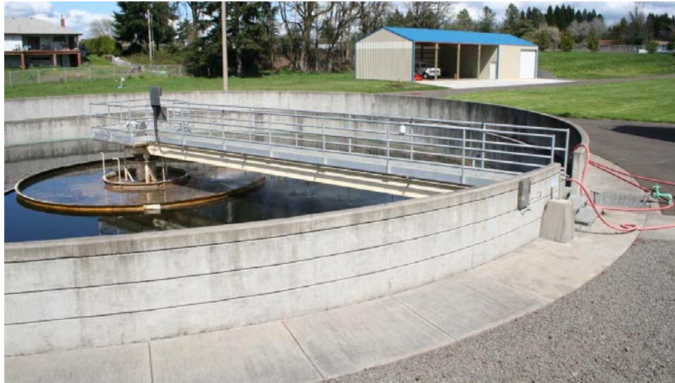
Figure 7-19: Silverton WWTP Secondary Clarifier
