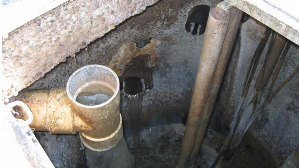
Figure 9-14: Manhole and Pump Station for Sidestream Recycle Flows
