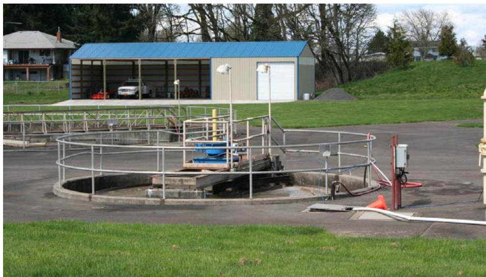
Figure 7-26: Silverton WWTP Primary Sludge Gravity Thickener
