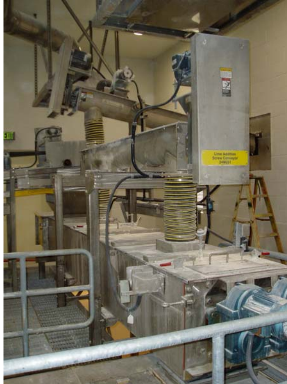
Figure 9-21: Lime Stabilization Facility in Newport, Oregon
