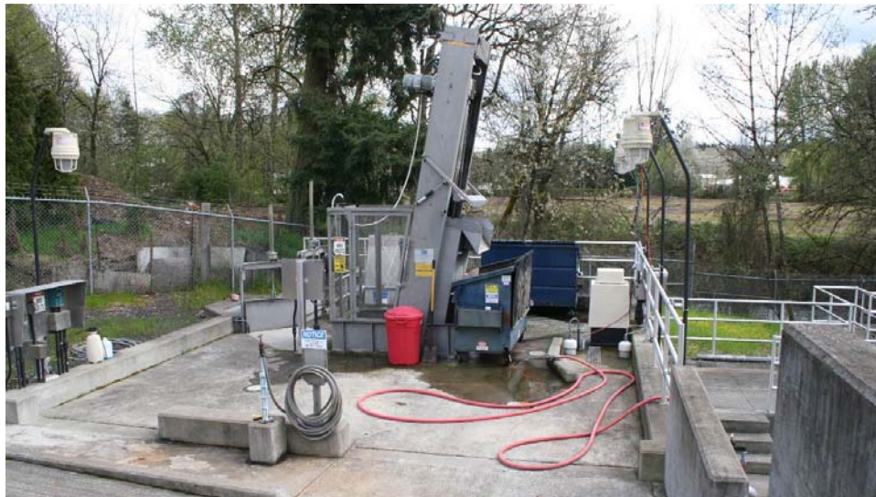
Figure 7-14: Silverton Headworks Single Bar Screen
