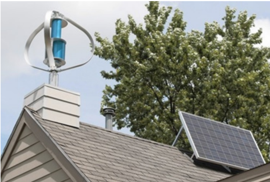
FIG NUM. 24 Rooftop wind turbine
