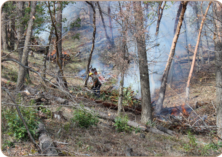
Above: Abraham Contracting crews pile burning on private lands in the neighborhood above Lithia Park, Ashland. Credit: Michael Coughlan
