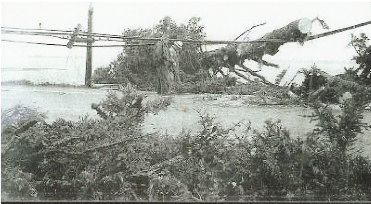
A TYPICAL SCENE IN MANY COASTAL AREAS ASSOCIATED WITH THE FEBRUARY 2002 STORM
