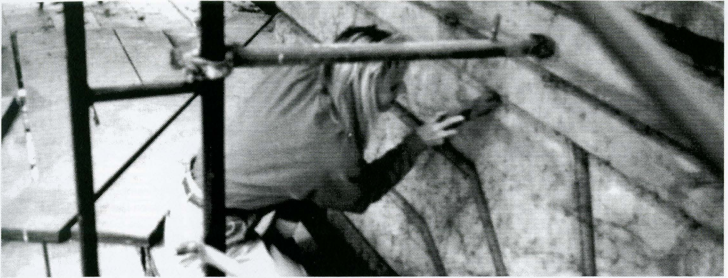
Kim Emerson, HP student working on the first phase of the Villard Hall roof and tower restoration project in the late 1980s
