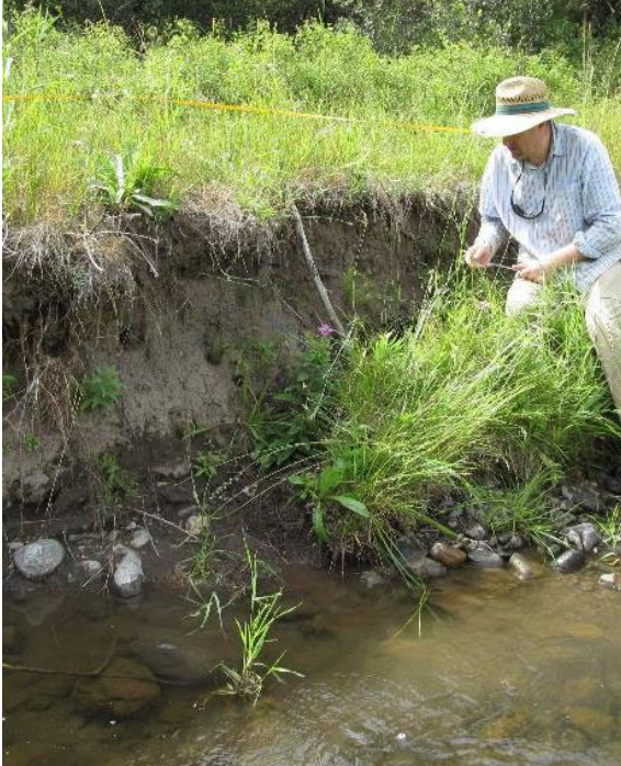
Figure 4.1. Cantilever failure block and composite bank. Note lower strata at left of photo with gravels and cobbles embedded in an eroding cohesive (sandy loam) matrix beneath upper cohesive strata.
