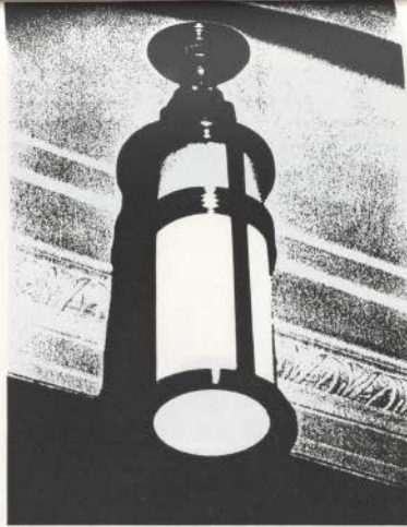
Figure 16. Stair lobby luminaire
