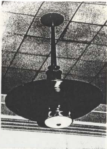
Figure 6. Second floor lobby luminaires
