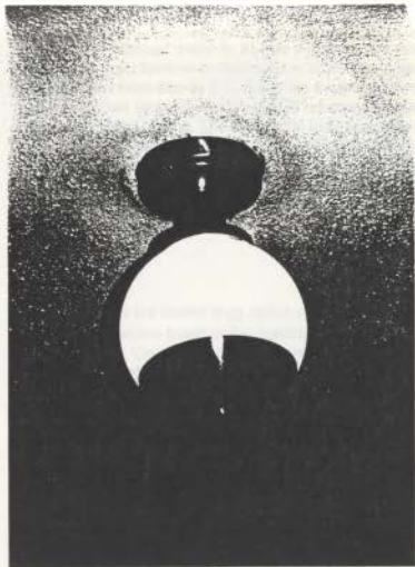
Figure 12. Third floor hallway luminaire
