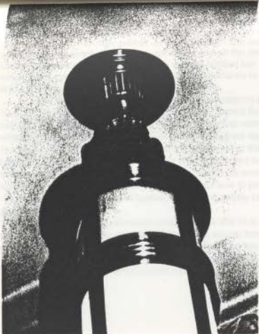
Figure 17. Detail of stair lobby luminaire
