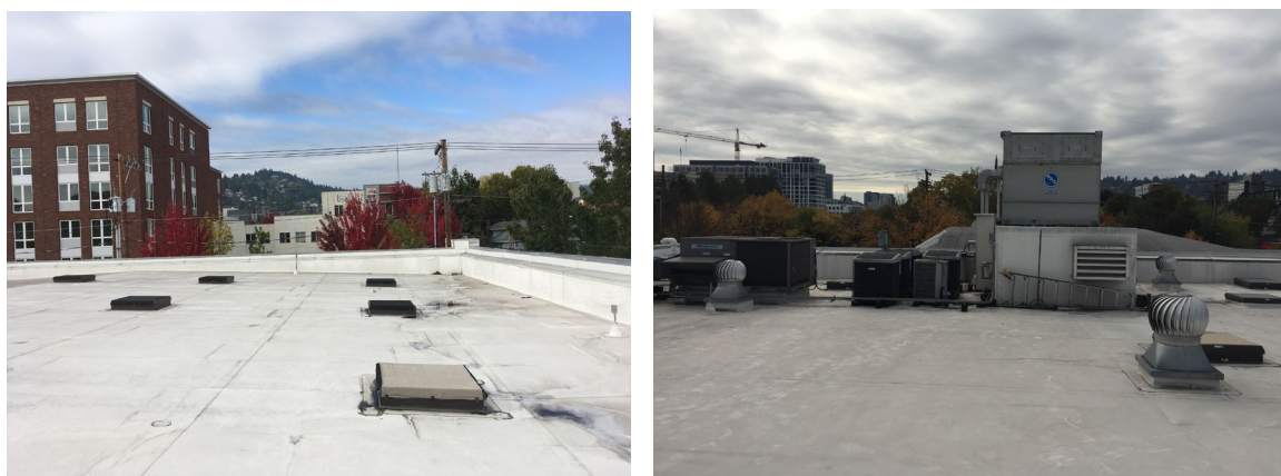
Figure 3: Exterior rooftop views: facing east (left) and facing south, showing roof vent and mechanical system (right). Source: (Marsie Surguine 2019)
