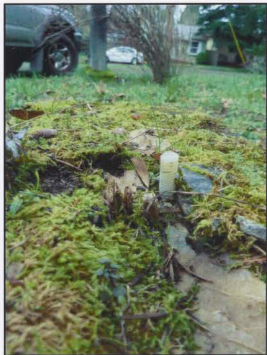
Detail of nylon pin, failed epoxy and mortar
