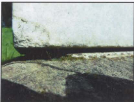
Deteriorated joint detail
