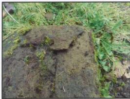
Detail of exfoliation and invasive root plant material
