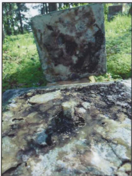
Detail of epoxy, mortar and pin at failed joint
