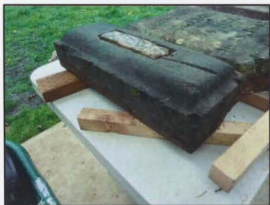
Transition element with broken marble portion
