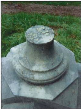
Detail of broken finial
