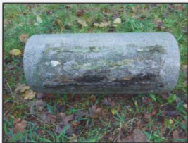
Detail of failed bonding material on granite element
