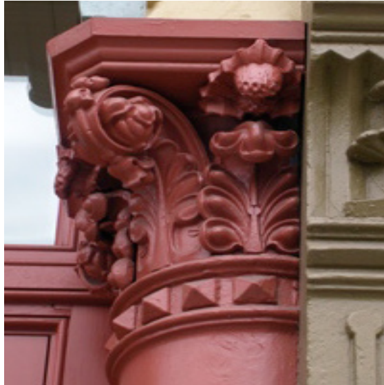
Figure 1. These cast iron columns and capitals on the east facing facade of the Bickel Block on NW Naito Parkway were re-cast in aluminum by Barr Casting in Portland after being discovered behind a brick wall. Photo: Bethany Johnson.
