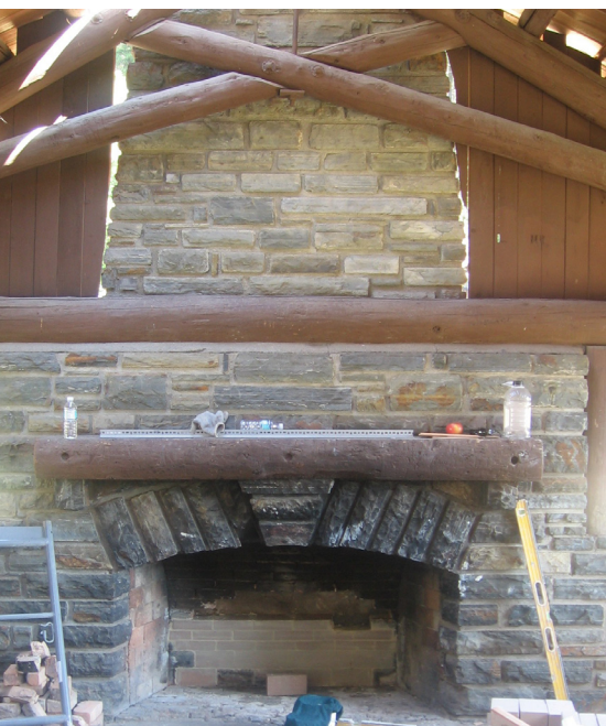
Figure 2. A view of the log scissor-trussed structural system and the massive stone fireplace with its segmental arched opening and heavy log mantel located on the northeastern end of the shelter. Photo: Abby Glanville.
