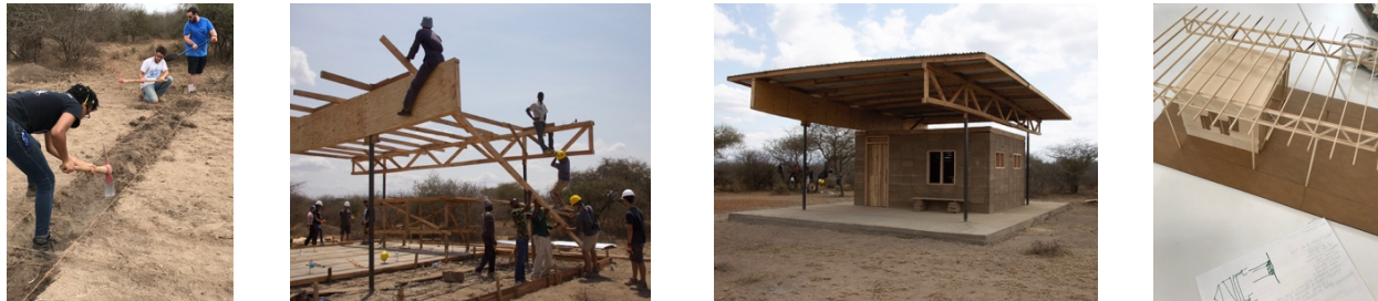
Figure 9. Trenching for grade beams; roof framing; finished structure; structural model made at University
