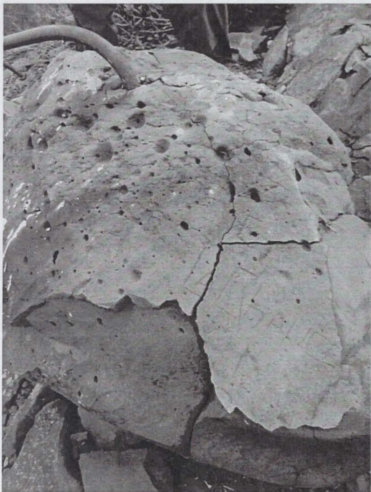
Figure 28. Northeast guy wire anchor at Frissell Point Lookout site; note paint, graffiti, and fire-damaged rock (photo by author, November 3, 2012).
