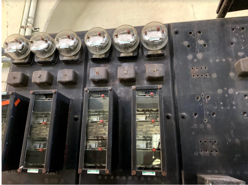
Figure C-37 Electrical board inside Bull Run Powerhouse. Source, author.
