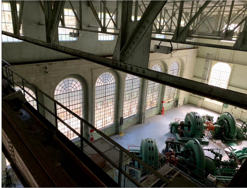
Figure C-27 Interior of Bull Run Powerhouse and generators from second story platform. Source, author.
