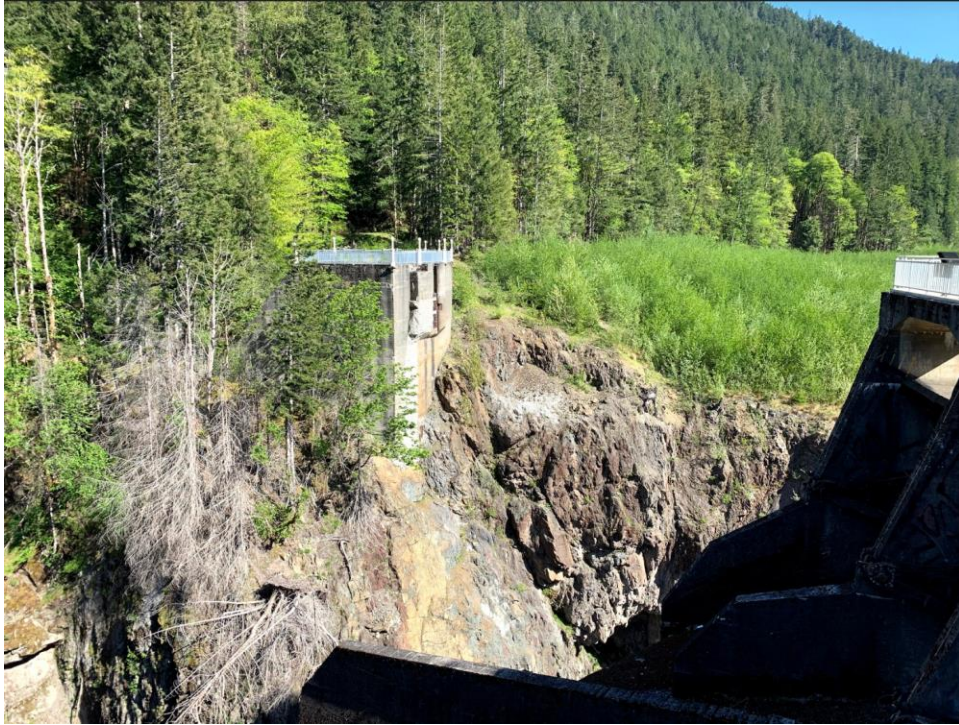
Figure C-58 Glines Canyon Spillway Overlook, view of preserved eastern wingwall and western spillway. Source, author.
