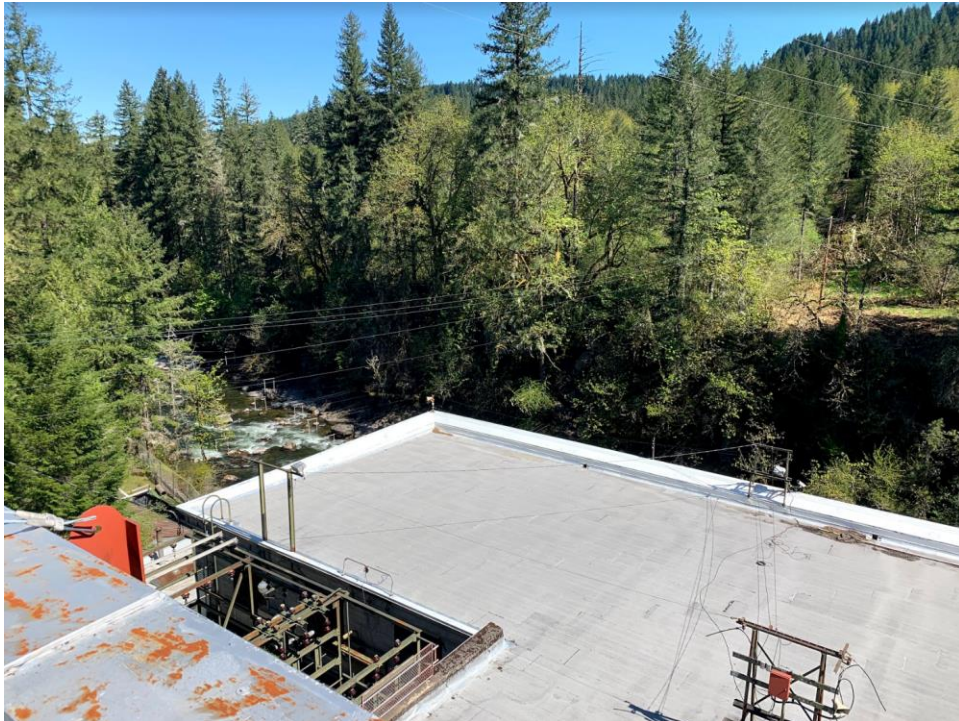
Figure C-30 View of Bull Run Powerhouse roof and Bull Run River from the roof of the Transmission Building. Source, author.
