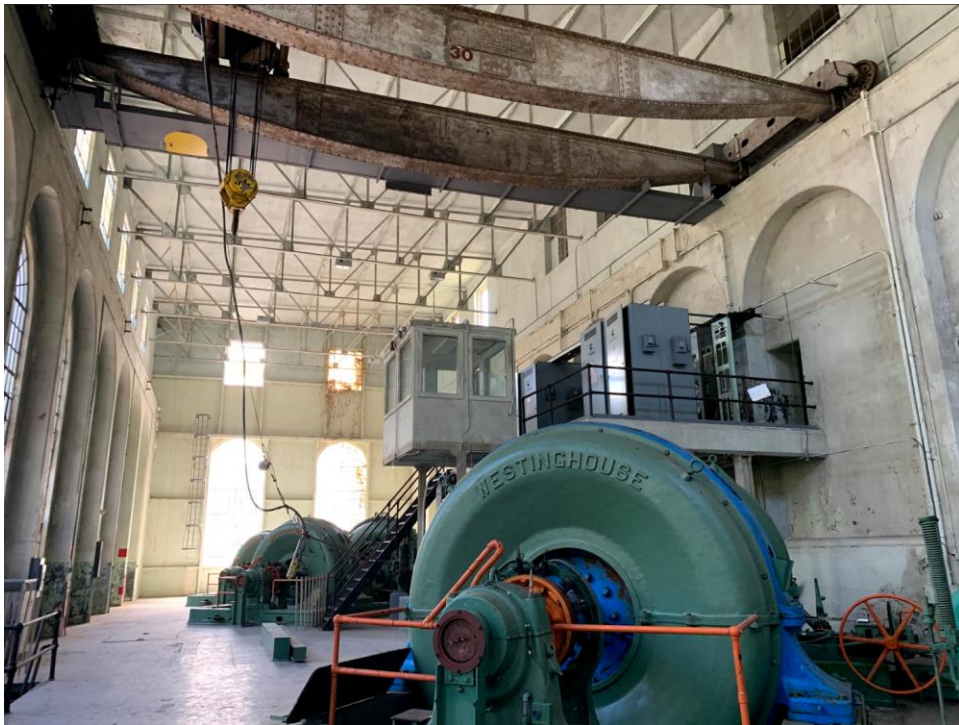
Figure C-34 Interior and generators of Bull Run Powerhouse. Source, author.
