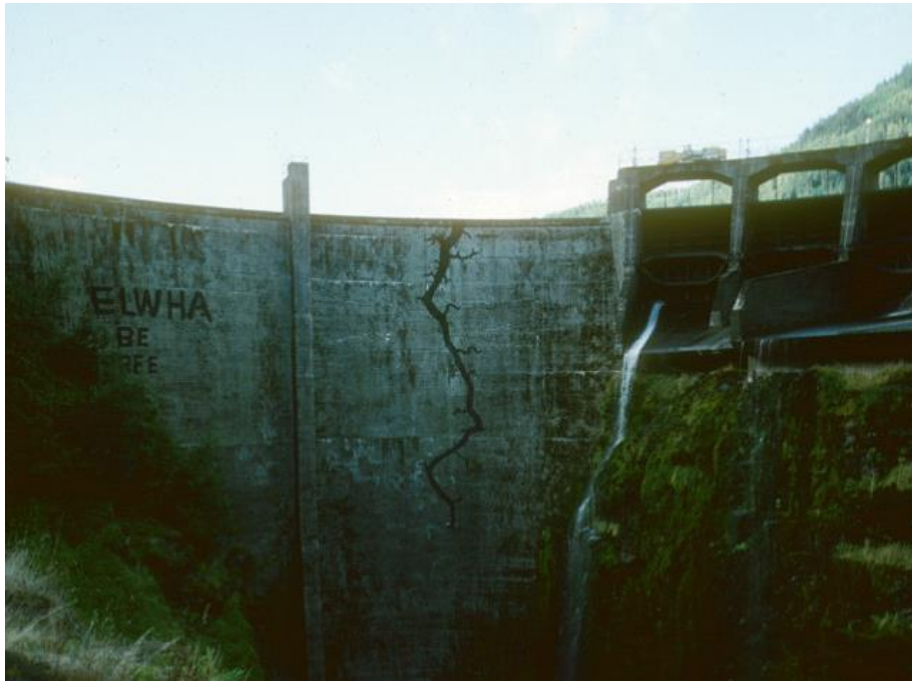
Figure 7.13 “ELWHA BE FREE” painted on the Glines Canyon Dam by Earth First!, 1986. Source, seattlemet.com .
