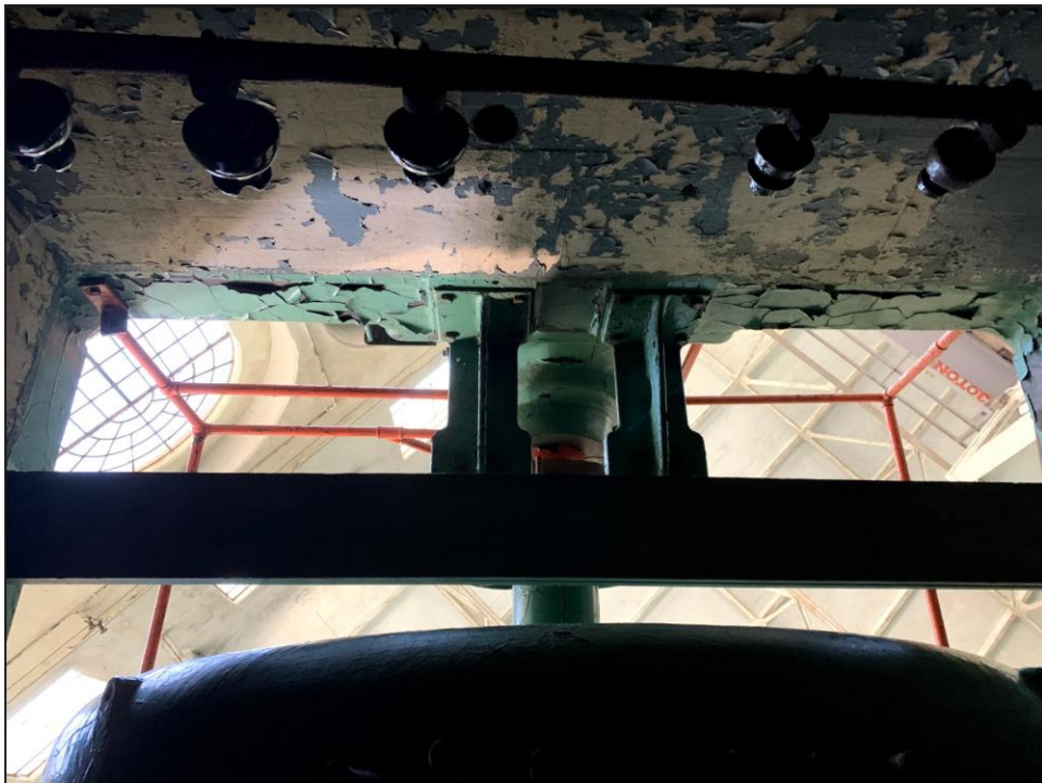
Figure C-36 View from below a generator in the Bull Run Powerhouse. Source, author.
