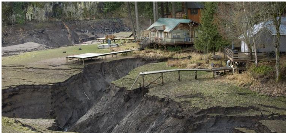
Figure 7.10 Erosion behind cabins located on the former Northwestern Lake, 2012. Source: The Columbia.
