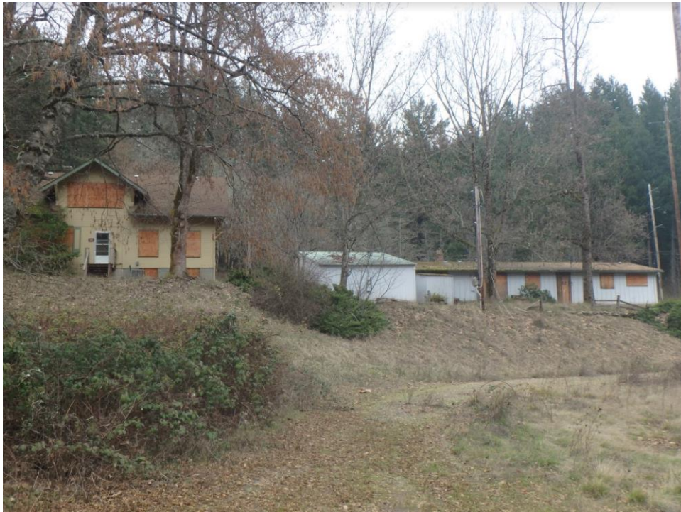
Figure C-6 Boarded up buildings at the Condit Hydroelectric Site. Source, author.
