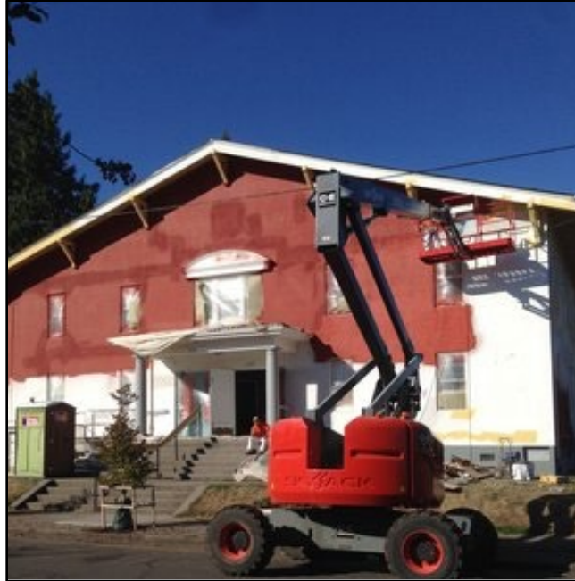
Figure 46. Painting the exterior of the building during renovation. Photo courtesy of Cerimon House.
