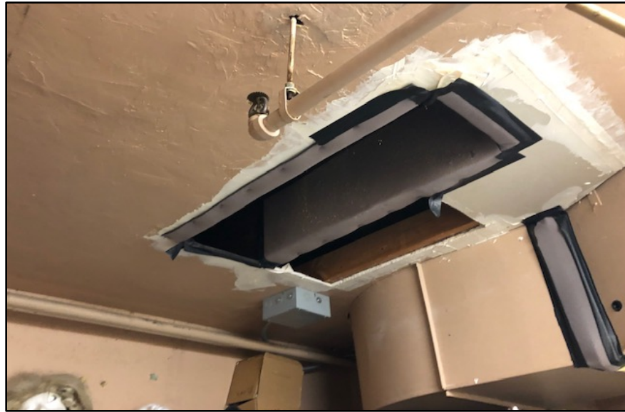
Figure 35. Trapdoor for auditorium found in basement of the building. Photo by author.
