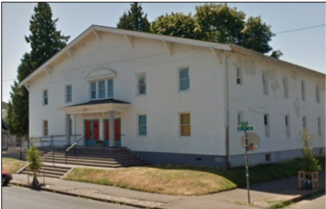
Figure 45. Photo showing building condition of Cerimon House one year after it was purchased during redevelopment. Noticeable areas where stucco has peeled off on north façade. Credit, Google Maps (2014).
