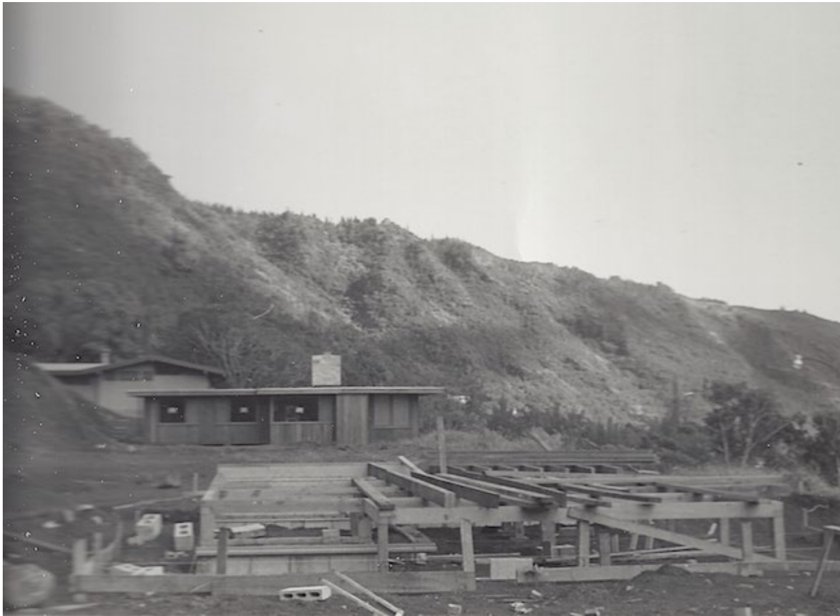
Figure 4.1 Construction phase of 3622 Woodlawn Terrace Place, southward view, 1956. Photo by Wallace Sanford. Courtesy of Claire Sanford.
