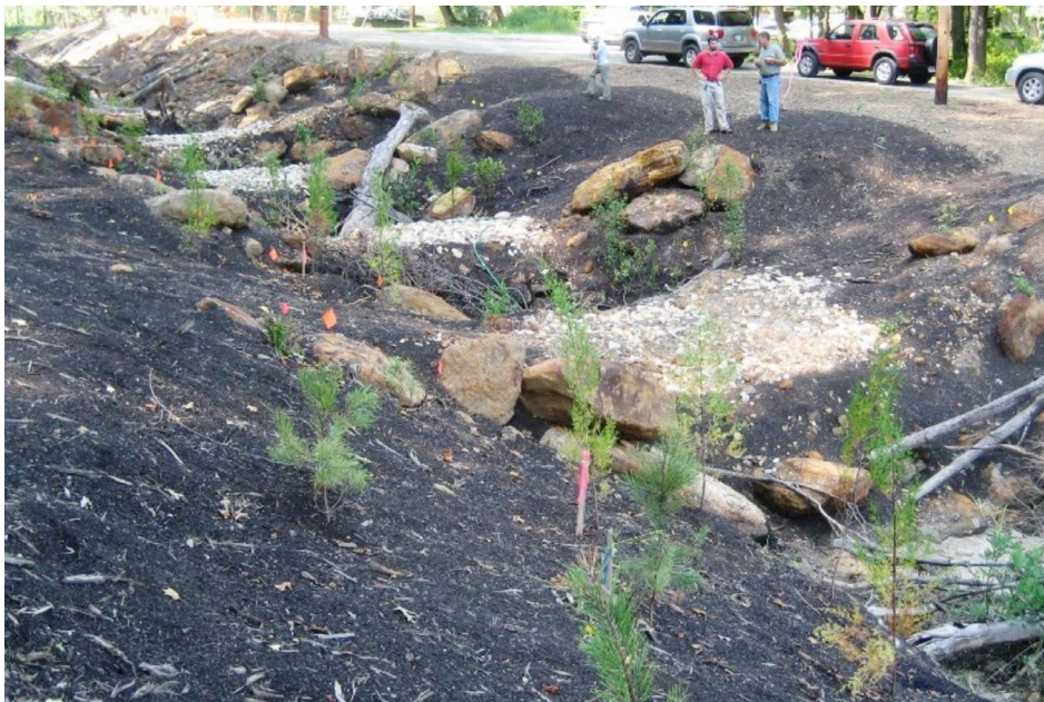
Figure 25: Phase 2 of Red Rock Creek enhancement. Examples of Grade Control. Source: Jennings Environmental LLC
