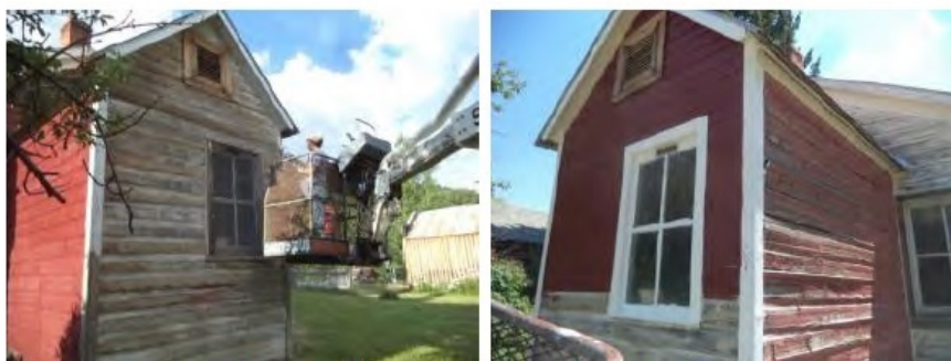
The north side is scraped, primed, and painted using the man lift.
