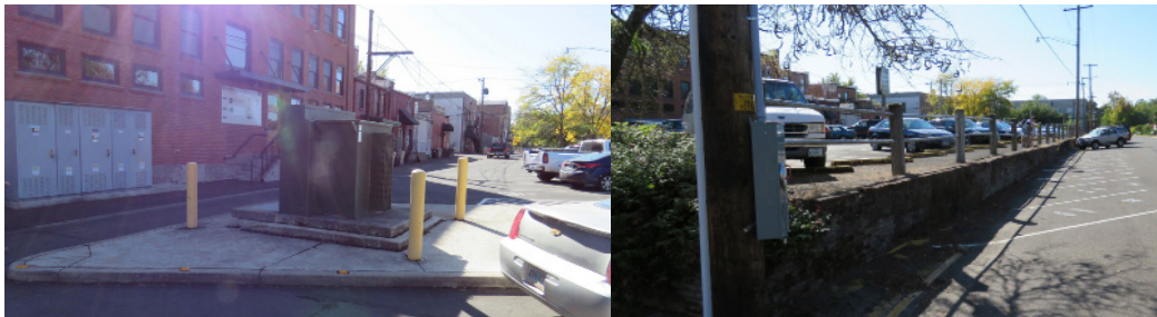
Transformer box on site
