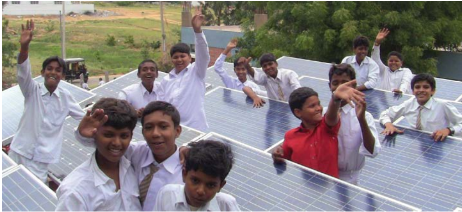
Students from the Jnana Bodhini School celebrate the installation of solar panels that help run their computer lab. Raj Vable, a graduate student in the UO environmental studies program, led the project.
