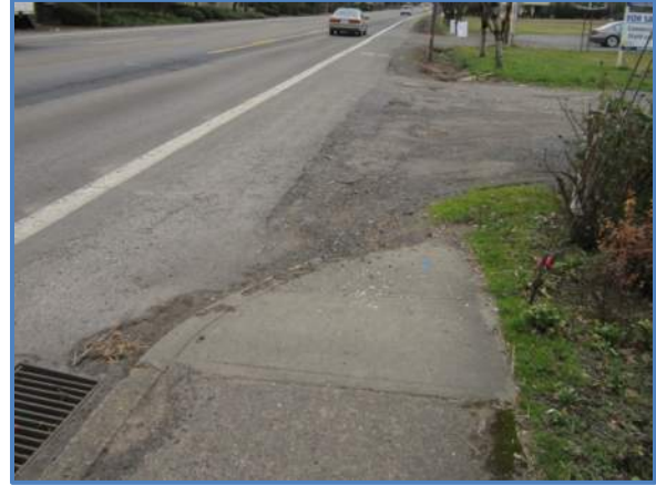
Curb ramp on 99W descending into deteriorated pavement
