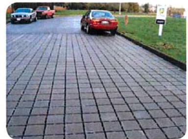
An example of permeable pavers
