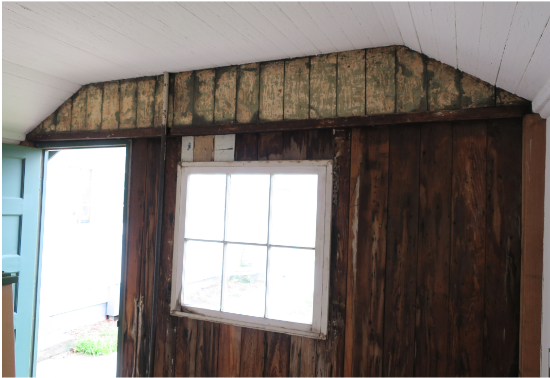
Figure 34: Newspaper wall lining is still visible in the Goldie Shacks. (Photo by author)
