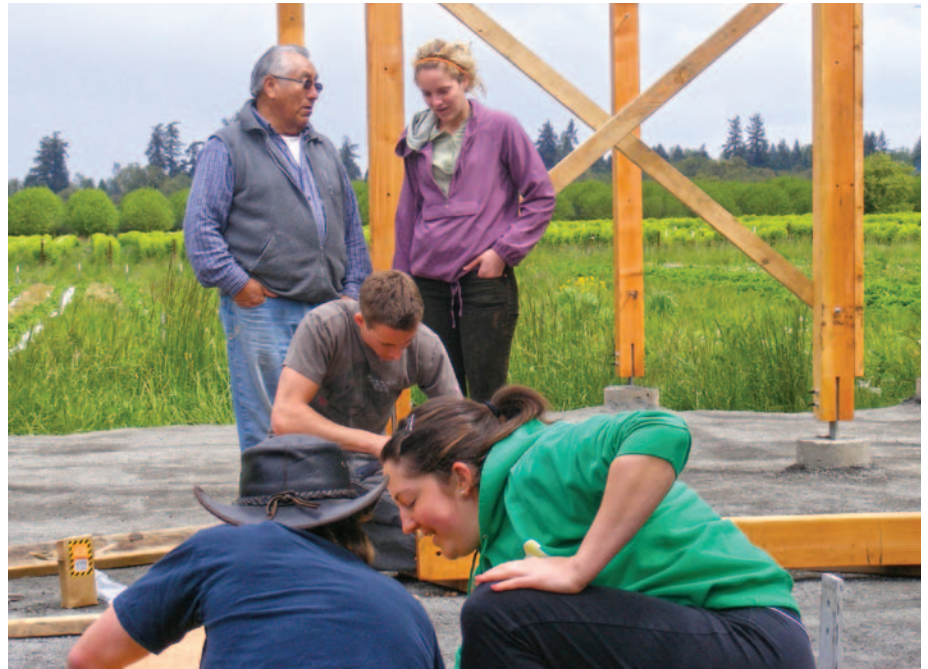
Acting Local Farmer Alberto Astuhuaman (in vest) watches UO designBridge students at work on Huerto de la Familia's multipurpose structure. DesignBridge is a multidisciplinary student organization linking the UO with the surrounding community by offering design and design-build services to local organizations that could most benefit from the help.
