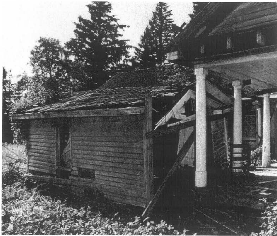
4.7 The house in the 1970s: the southwest corner of the porch, with the ruinous wash house near collapse.
