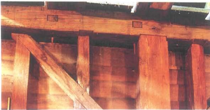
3.5 The woodshed, the north wall. The rectangular sockets--mortises--in the plate suggest that the piece was salvaged material, probably from a barn.
