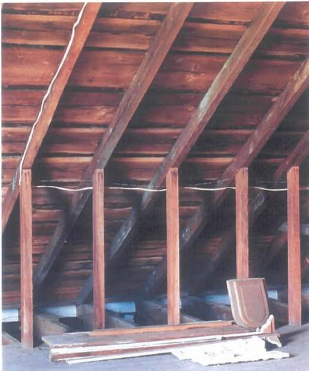
3.11 The attic. The taper of the rafters, from eave to ridge, can just be discerned. The colonnade outriggers are visible beyond the vertical members that rise from the exterior wall below.
