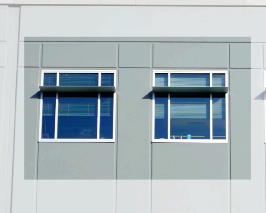
Figure 16: Typical fenestration design for windows on the first, second, and third floors showing divided lites and exterior horizontal shading surface.
