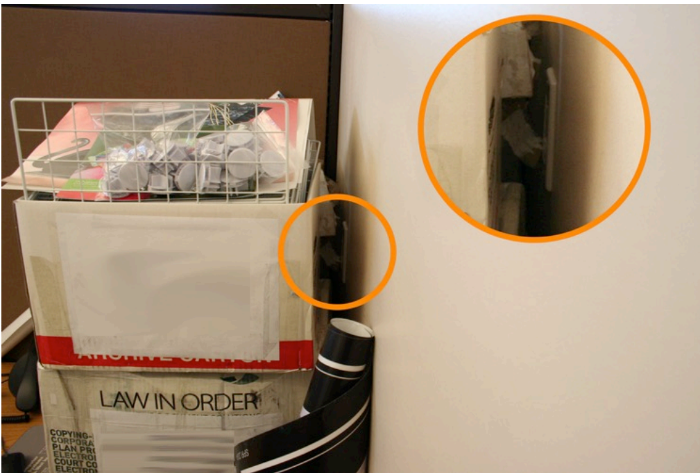
Figure 152: Corridor and office lighting control in office #112 completely blocked by occupant's storage boxes.
