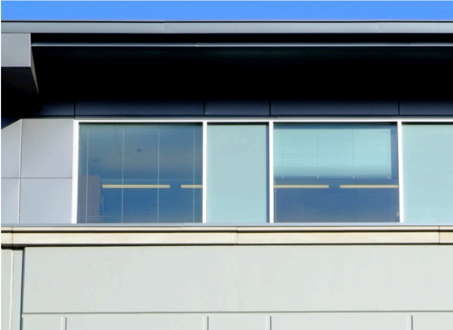
Figure 17: Typical fenestration design for windows on the fourth floor showing alternating pattern of clear and opaque lites within the structural bay and roof overhang above.
