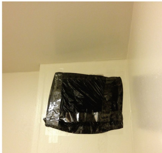
Sealed Bathroom Vent
