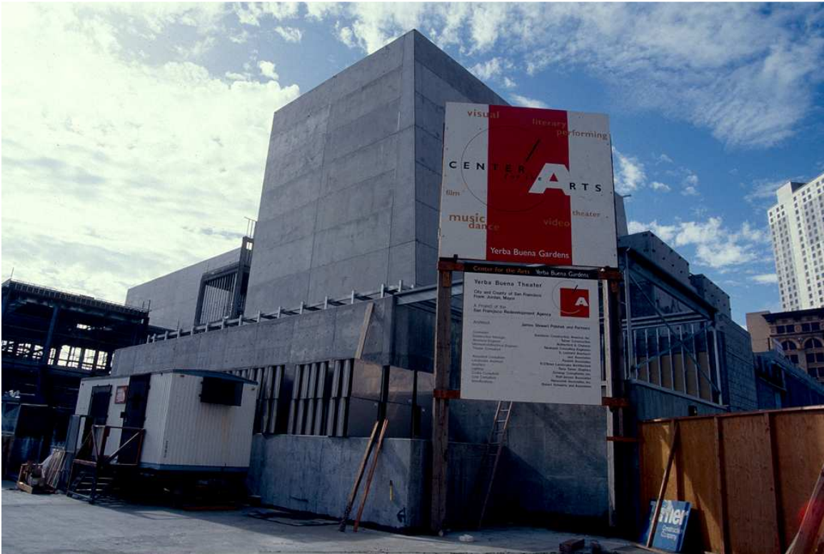
Fig. 8. Construction of the Yerba Buena Center for the Arts, 1992, San Francisco. Photographs courtesy of the Yerba Buena Center for the Arts.
