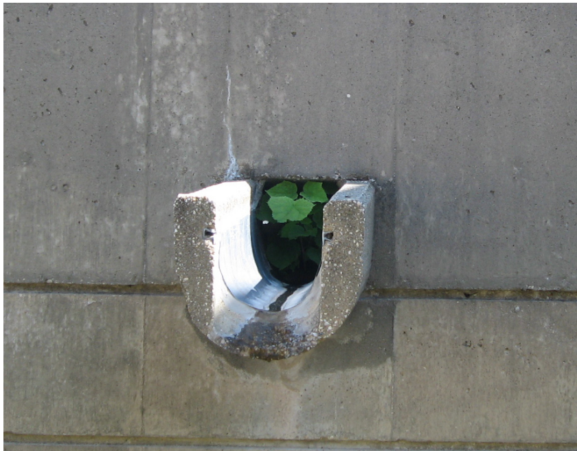
Figure 39 - Organic growth in the gutter
