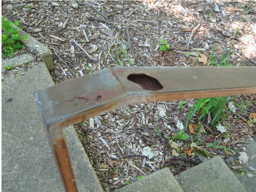
Figure 38 - Corrosion on metal rail
