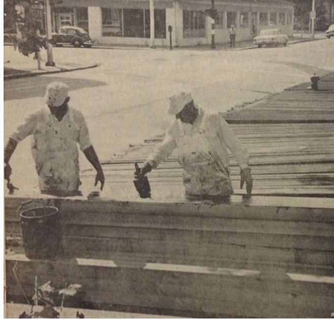
Figure 3.4. Staining the 800 vertical cedar slats for the wood screen, 1963. Image source: Eugene Register Guard .
