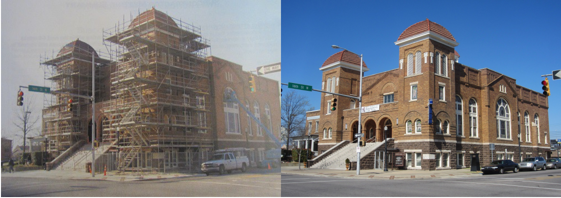
Church mid-preservation, looking Northwest (early 2007, courtesy of Architecture Works/ March 20, 2014, courtesy of author)
