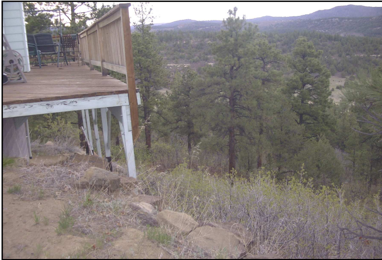
Heavy fuel on slope below this structure make it unlikely that the structure will survive a wildfire
