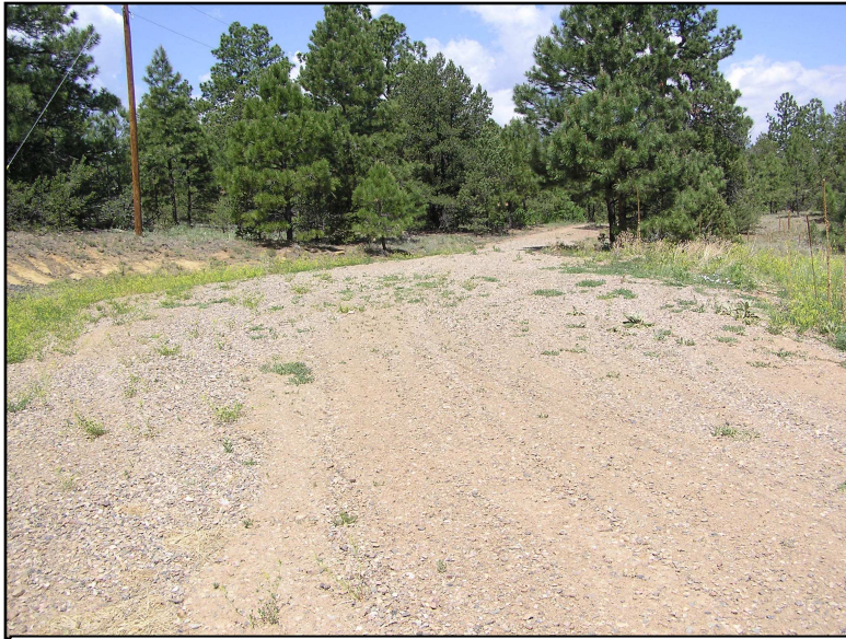
Inadequate turn radius at the end of Spirit Mountain Place
