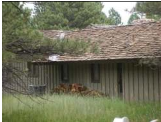
Figure 26. Significant combustible exterior fuel loads
