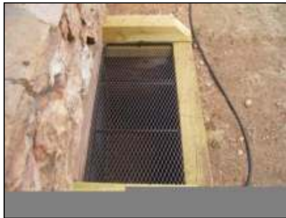
Figure 28. Window wells collect should be screened
