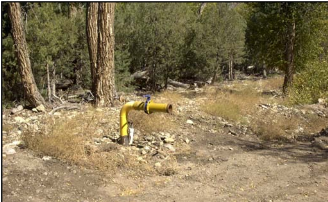
Dry hydrant and 6,000 gallon fire cistern located on Zapata Creek in Zapata Subdivision
