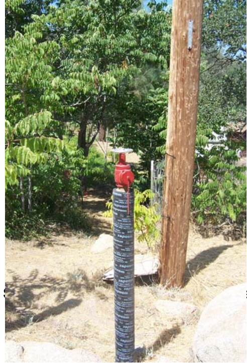
Standpipe in 700 block of South Alpine
