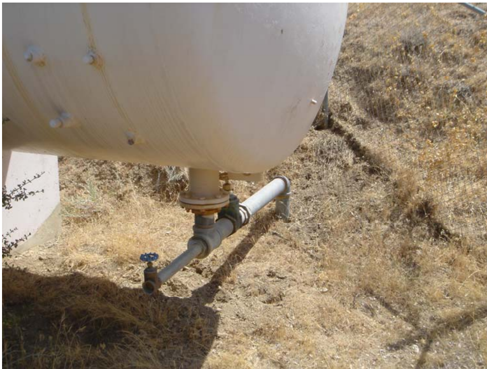
View of 2" IPF valve under water tank on the south end of the tank
