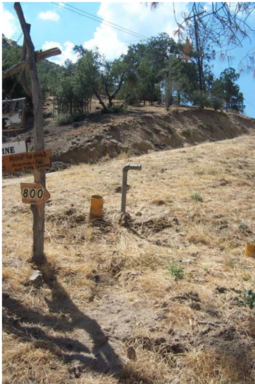
Standpipe in 800 block of South Alpine
