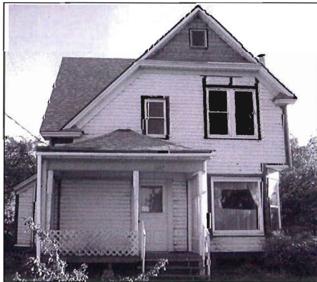
During rehabilitation, the incompatible metal siding was removed, and original wood siding exposed and restored. Paint lines indicate location of original trim
