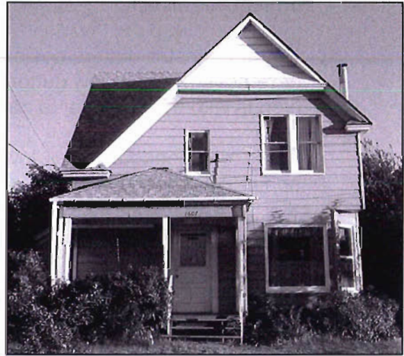
Wide metal siding replaced original narrower horizontal wood siding and original door and window trim were removed in 1970s. The loss of historic material and integrity is evident
