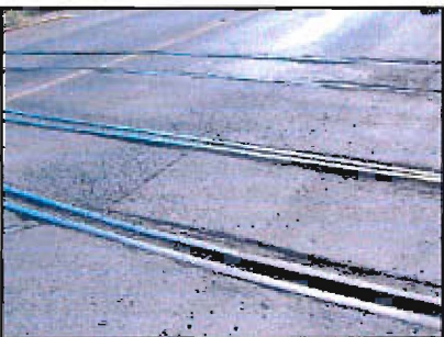
Existing railroad tracks that cross 5th Avenue present a hazard for cyclists
