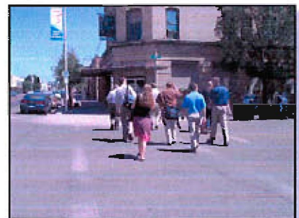
Faded crosswalk exist at several downtown intersections
