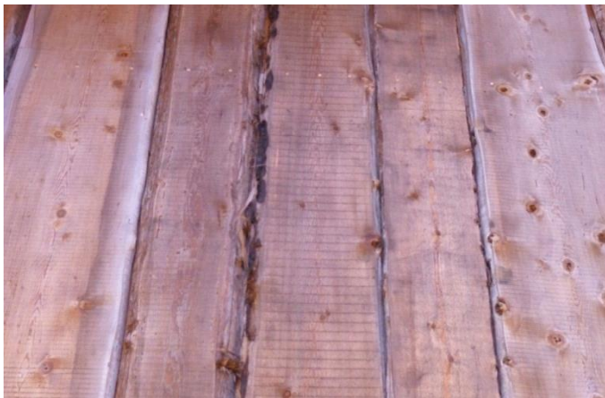
Figure 10. Detail of wood plank wall. Note row of wood peg fasteners near the top ( photo by author ).
