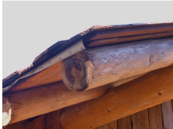
Figure 11. View of roof structure. Note layers of plywood and water-resistant material ( photo by author ).
