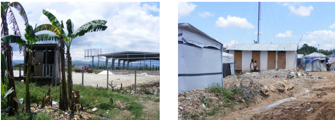
Figure 5.39. Photographs of latrines in PDS. Left: Latrine in Sugar Canaan, which has become unusable since an aid organization stopped maintaining it. Around one hundred families share this latrine. Right: A latrine in Save the Children that is maintained by an aid organization. Photos by author.
