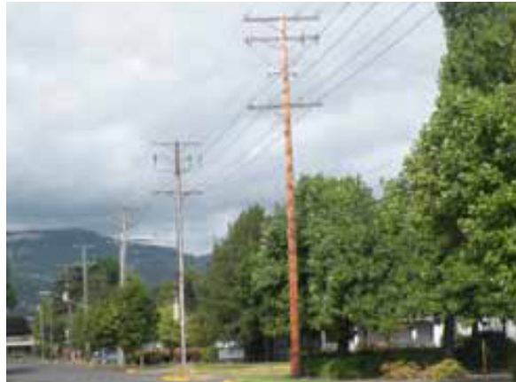
Figure 25: Power lines along 16th Street.
