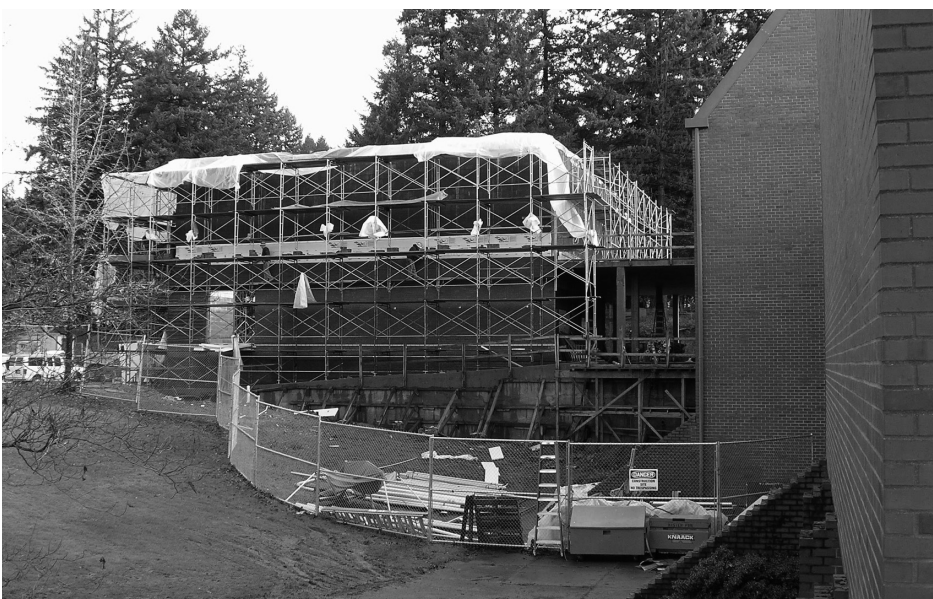
The Thelma Schnitzer Performance Wing is located at the northeast corner of the current music building. It will house jazz and percussion studies, a new large rehearsal room, classrooms, and a new recording studio.
