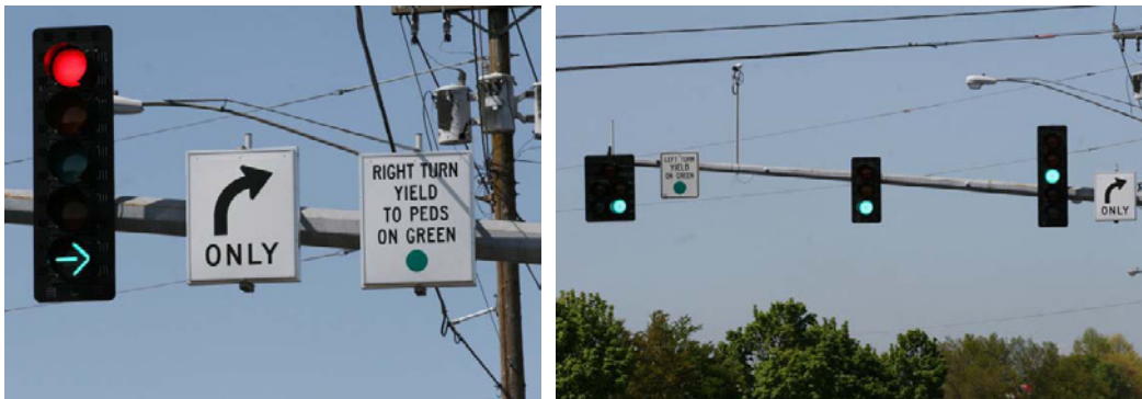
Figure 40: Traffic signals at intersection.
