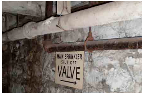
c) basement sprinklers
